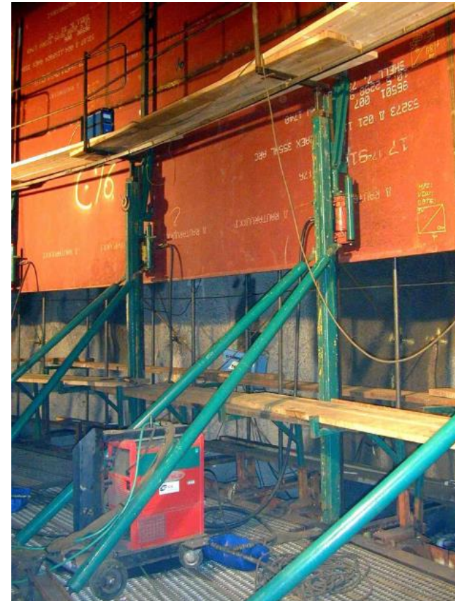
Lined cavern under construction for Natural Gas (Source: Thermie B - Project N° OG./270/97/SE/FR)
