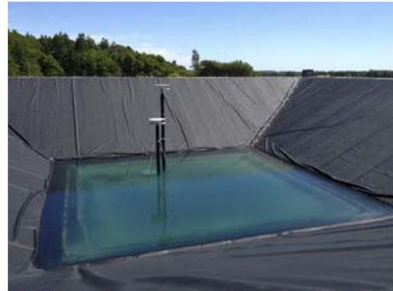
Figure 4.1 Picture of Dronninglund Pit Storage under construction. Dronninglund District heating; 37,573 m 2 of solar collectors and a 62,000 m 3 water in pit heat storage (PlanEnergi)
