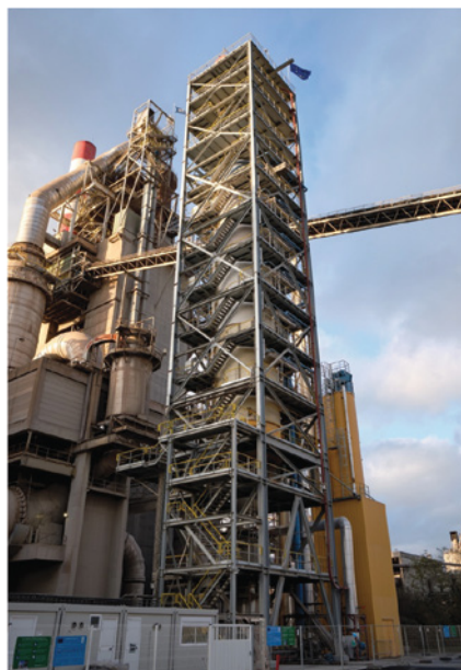
Figure 2: LEILAC1 Pilot Plant
